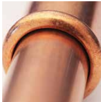
Unpressed fitting - small gap between fitting and tube.
