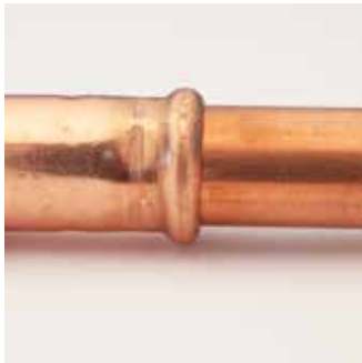
Pressed fitting - indents on fitting.
